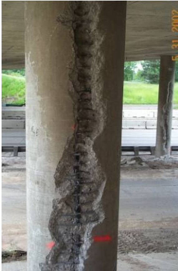
Figure 3.5: Column Damage Due to Explosion under Bridge. (Bridge Removals, FHWA)
