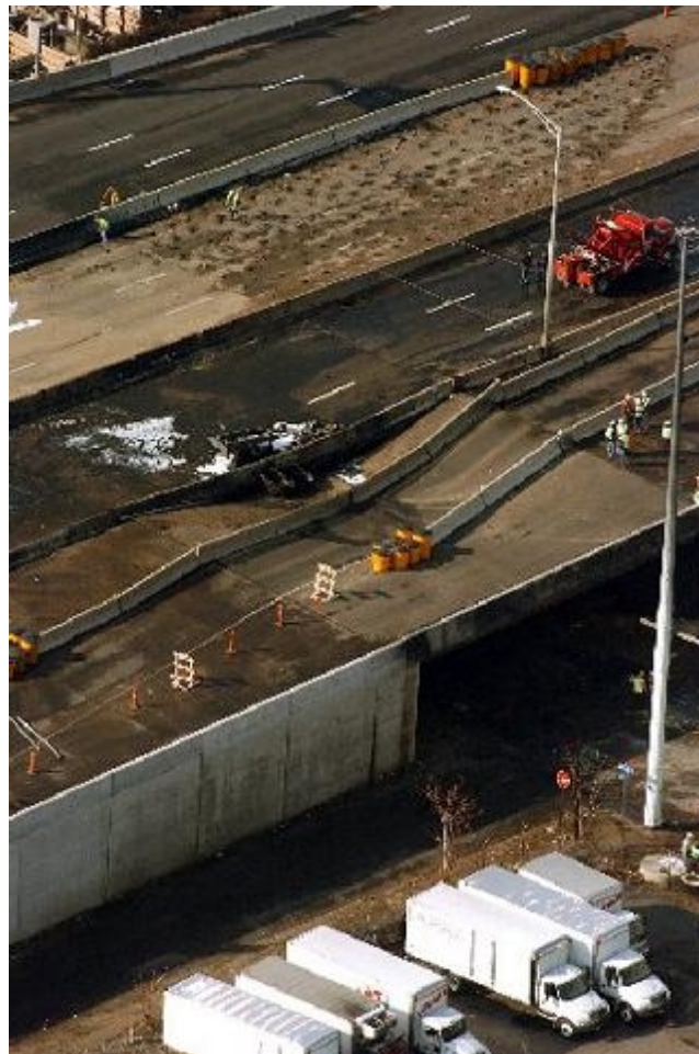
Figure 2.2: Oil-Tanker Burned on Interstate 95. (AP, Connecticut Post, March 2004)
